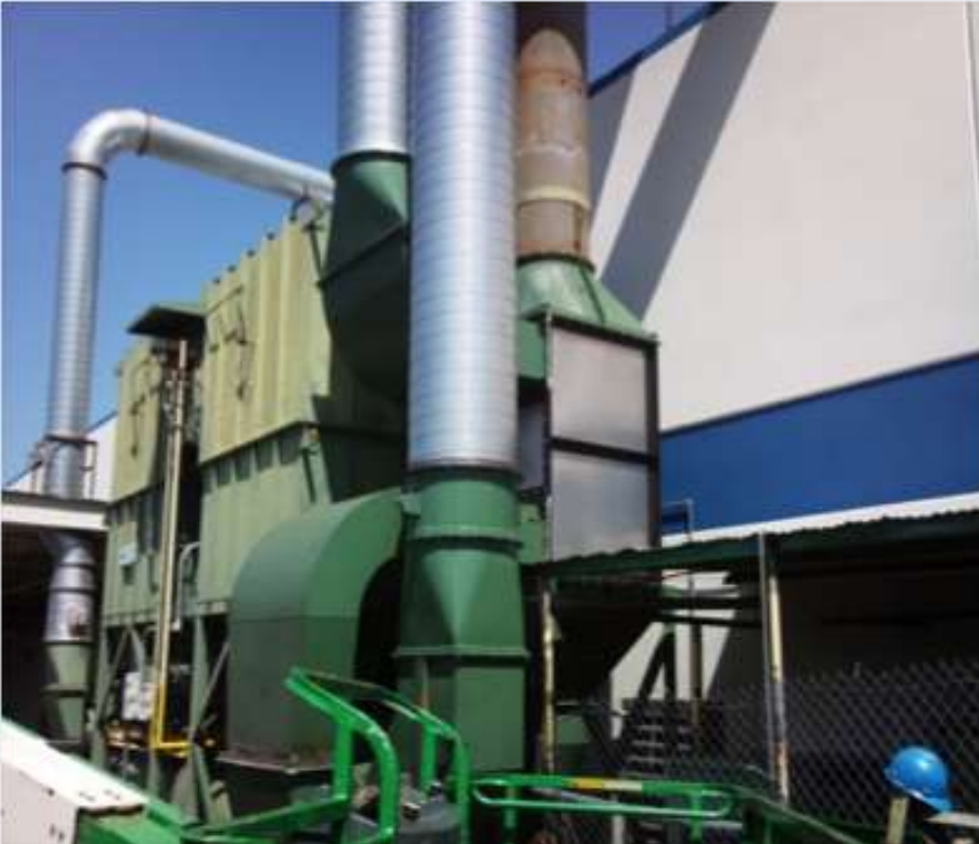
Heat Exchanger Installed on RTO Exhaust Stack to Capture Waste Heat & Provide Warm Process Air
