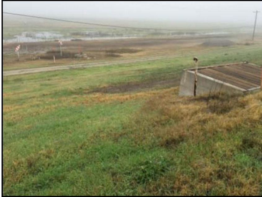
Figure 4. View of North Slope of Levee at North Landing. Pipeline Vault at Right.
