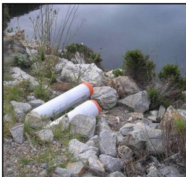
Figure 2-5. Existing Onshore Cable Conduits
